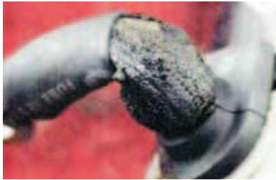
Strap damaged from heat
